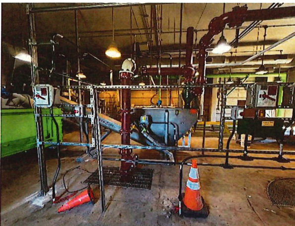
Figure 3: Grit Removal System Startup
